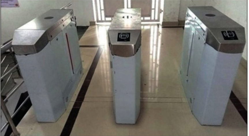
SECURITY CHECK: Automatic entry gate system has been installed at the entrance and on different floors of LU's Tagore Library
